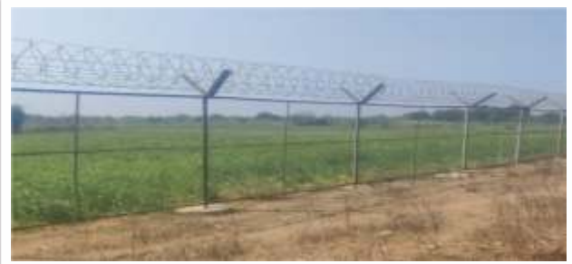
Boundary Fencing at Jhansi Solar Park
